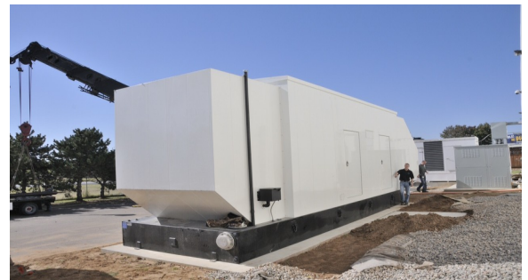
New 2 MW Sound Attenuated Walk -In Generator in Oklahoma City provided by Atlantic Controls and Hennig Enclosure Systems
